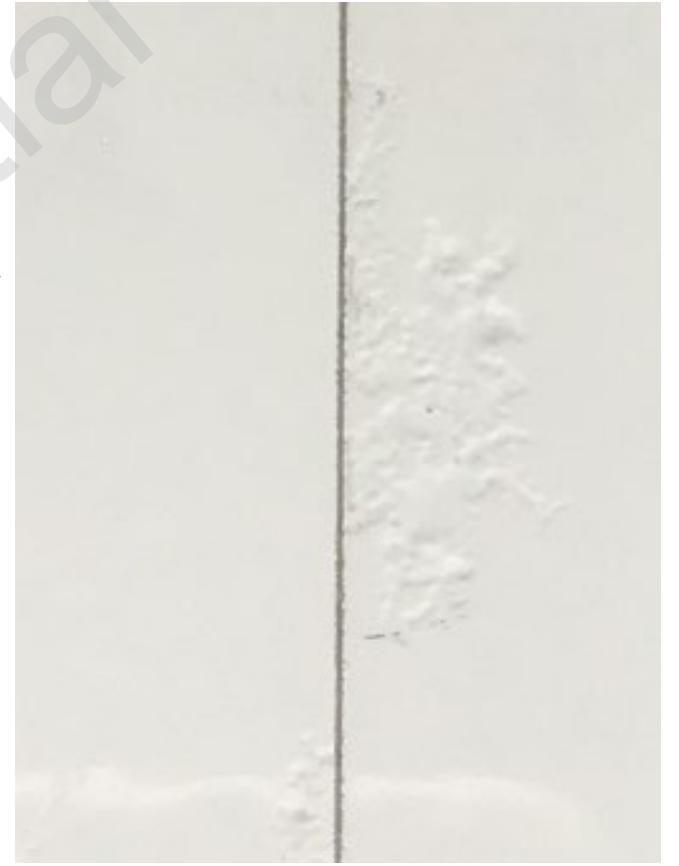
Corrosion morphology – Type B 腐蚀形貌 – 类型B
