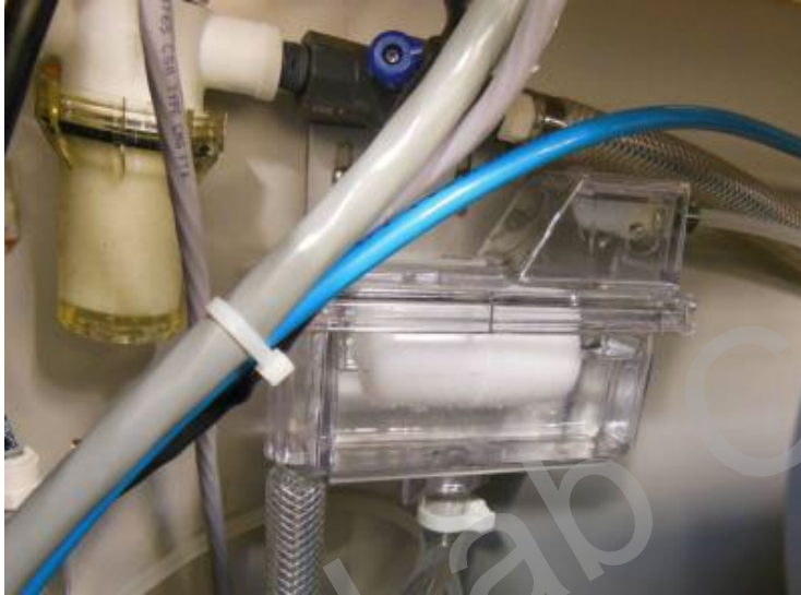
Water Feed Box (supply for wet bulb/dry bulb)
