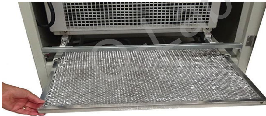
Chiller Air Filter
