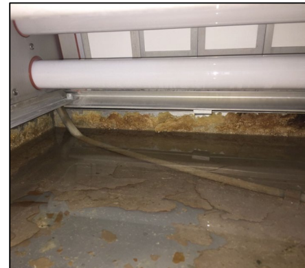
Significant mineral build-up
