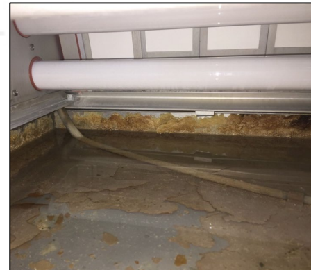
Significant mineral build-up
