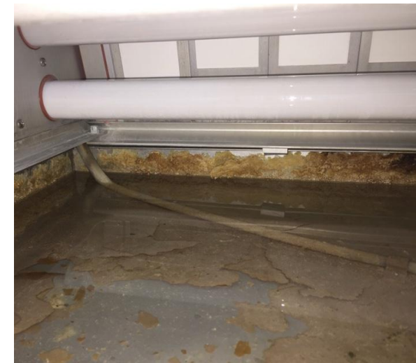
Significant mineral build-up
